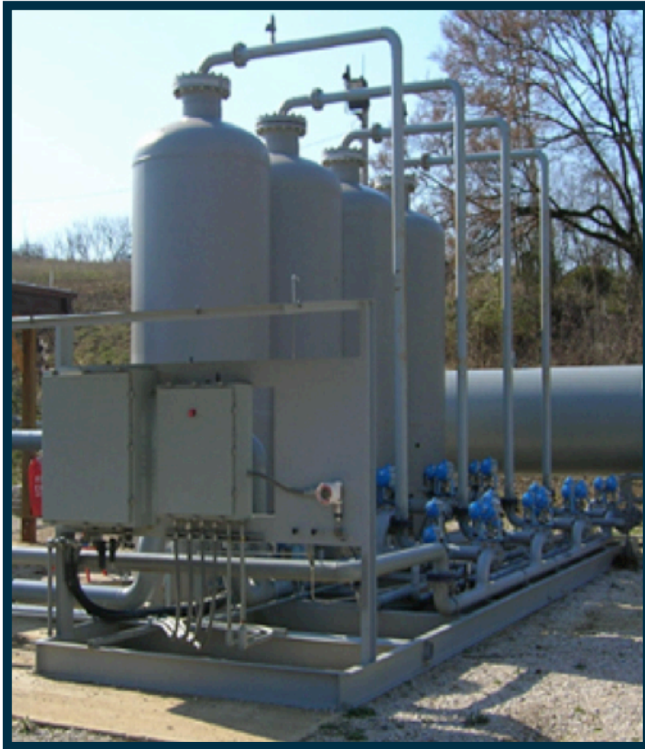
Figure 1-12: Natural gas dehydrator unit 62
