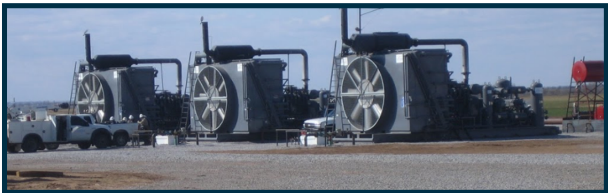
Figure 1-14: Natural gas compressors 65
