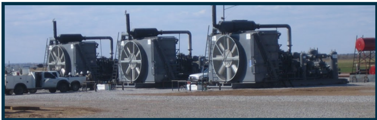
Figure 1-14: Natural gas compressors 65
