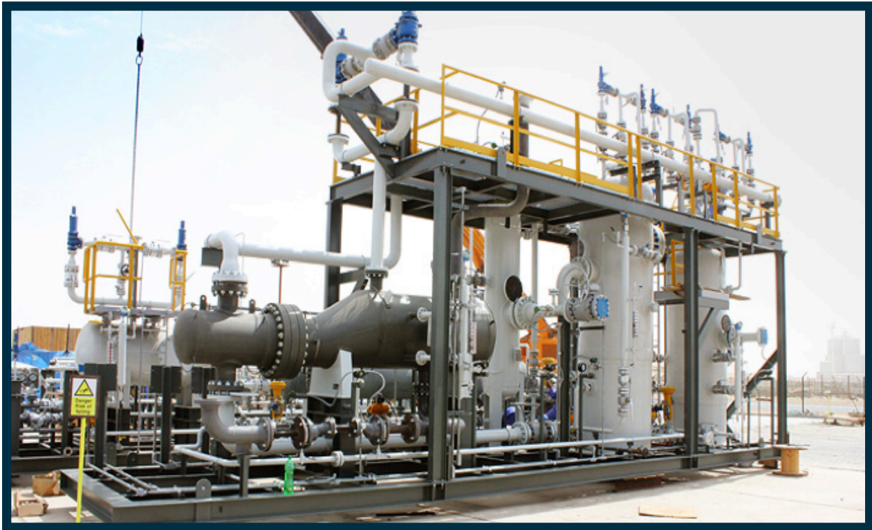
Figure 1-13: Natural gas sweetening unit 63
