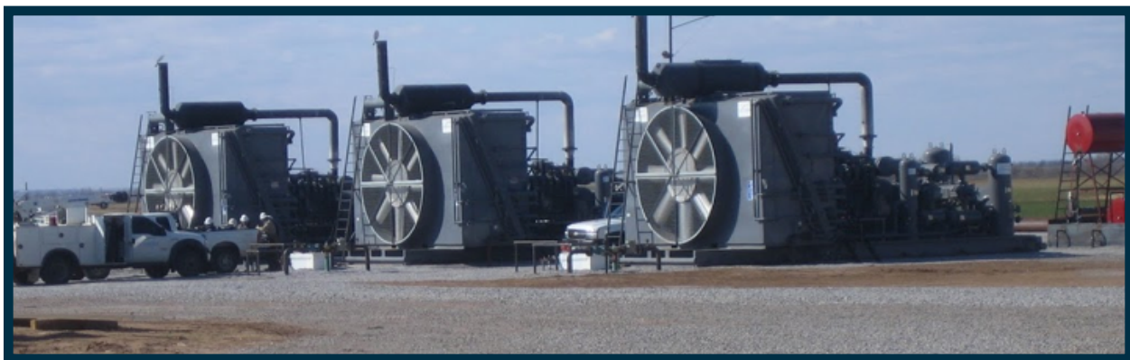
Figure 1-14: Natural gas compressors 65
