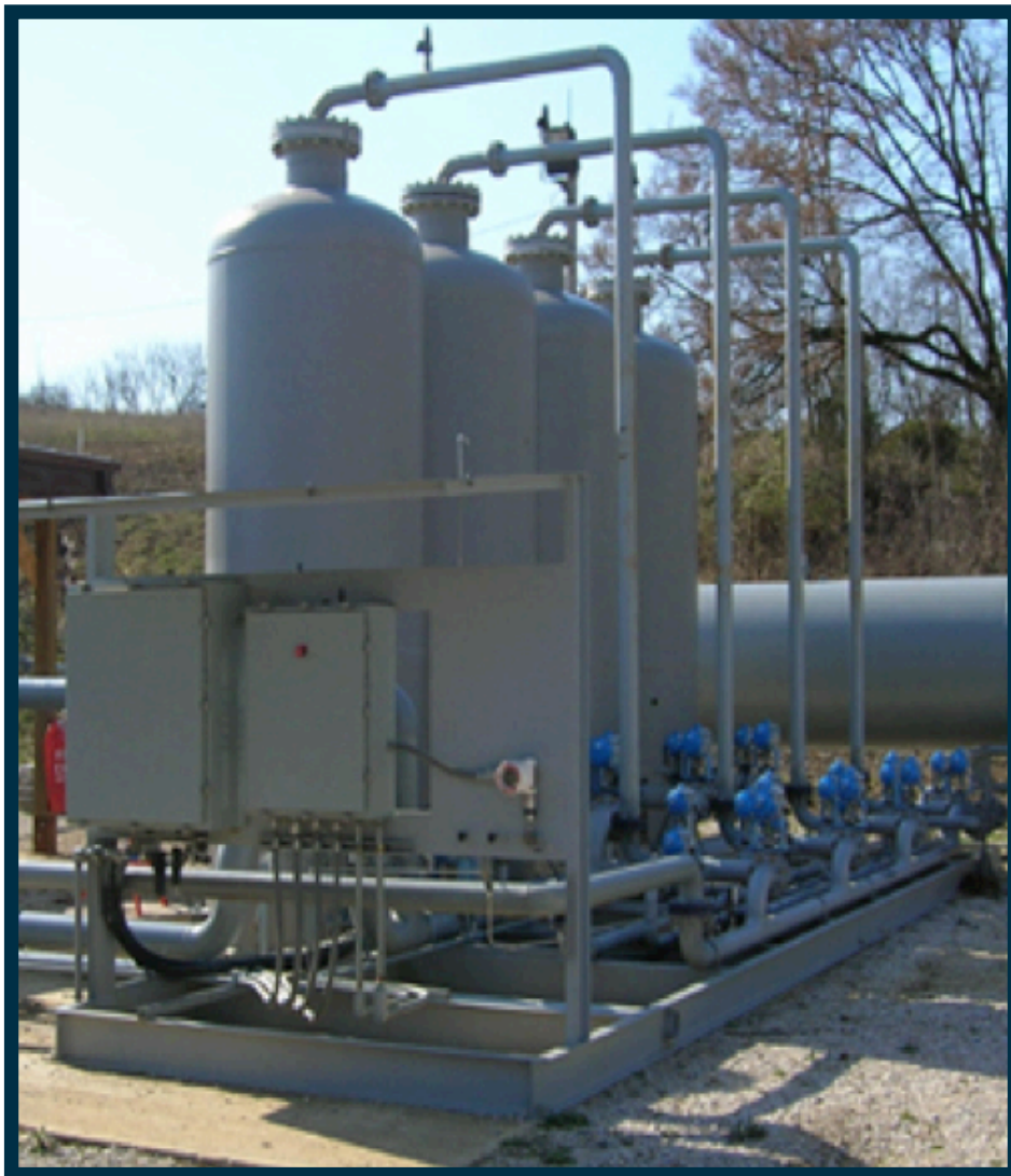
Figure 1-12: Natural gas dehydrator unit 62
